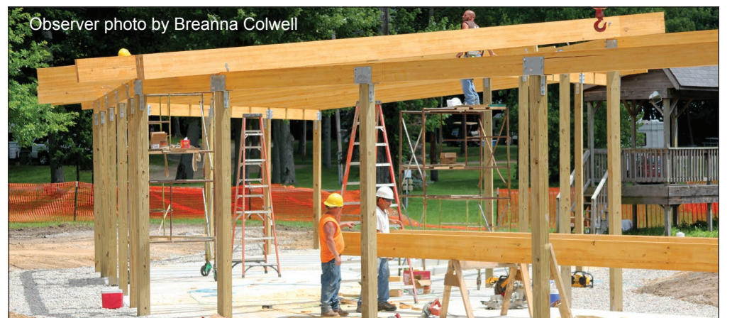
Observer photo by Breaonna Colwell The construction of the permanent pavilion on the "Hill." The newly renovated design of the pavilions will provide shade, shelter and seating from the sun and rain.
